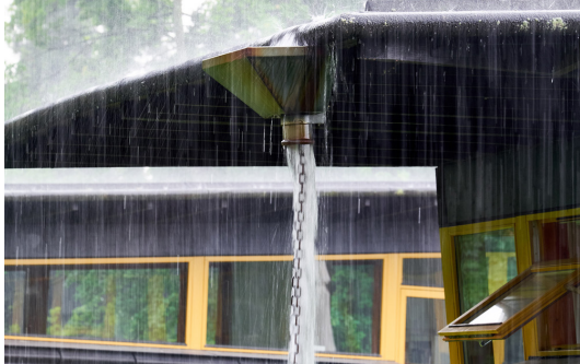
Roof Scupper Waterfall
